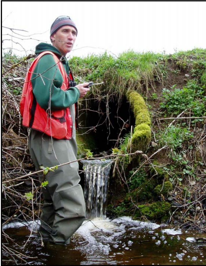
Figure 35. Michelena Creek perched SR 112 culvert.
