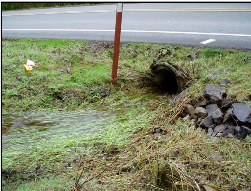
Figure 28. Razz Creek Tributary 1, looking downstream at SR 112 culvert where stream flows across highway during high flows.
