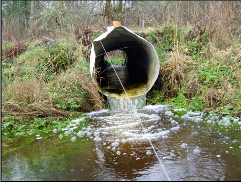
Figure 23. Perched culvert acting as a partial barrier to juvenile salmonids at the W3000 Road crossing.
