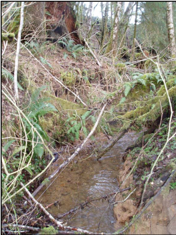
Figure 49. Razz Creek Segment 5, photo depicting channel incision in the upper half of Segment 5.
