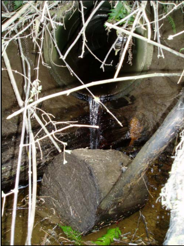
Figure 22. Perched culvert limiting fish access and tidal exchange in Section 9 Tributary (Farm Road crossing).
