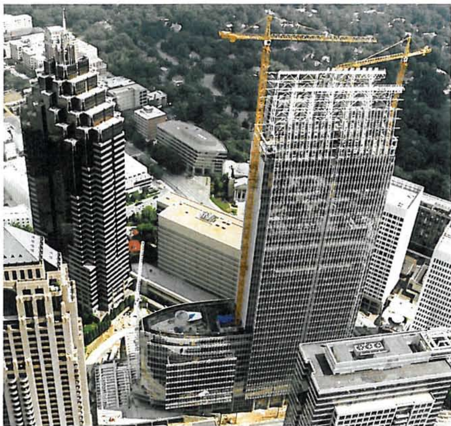
The structure will include a 119-ft.-tall lighted veil at its top. (Photo courtesy of Aerial Innovations of Georgia/www.aerialinnovationsofga.com)
