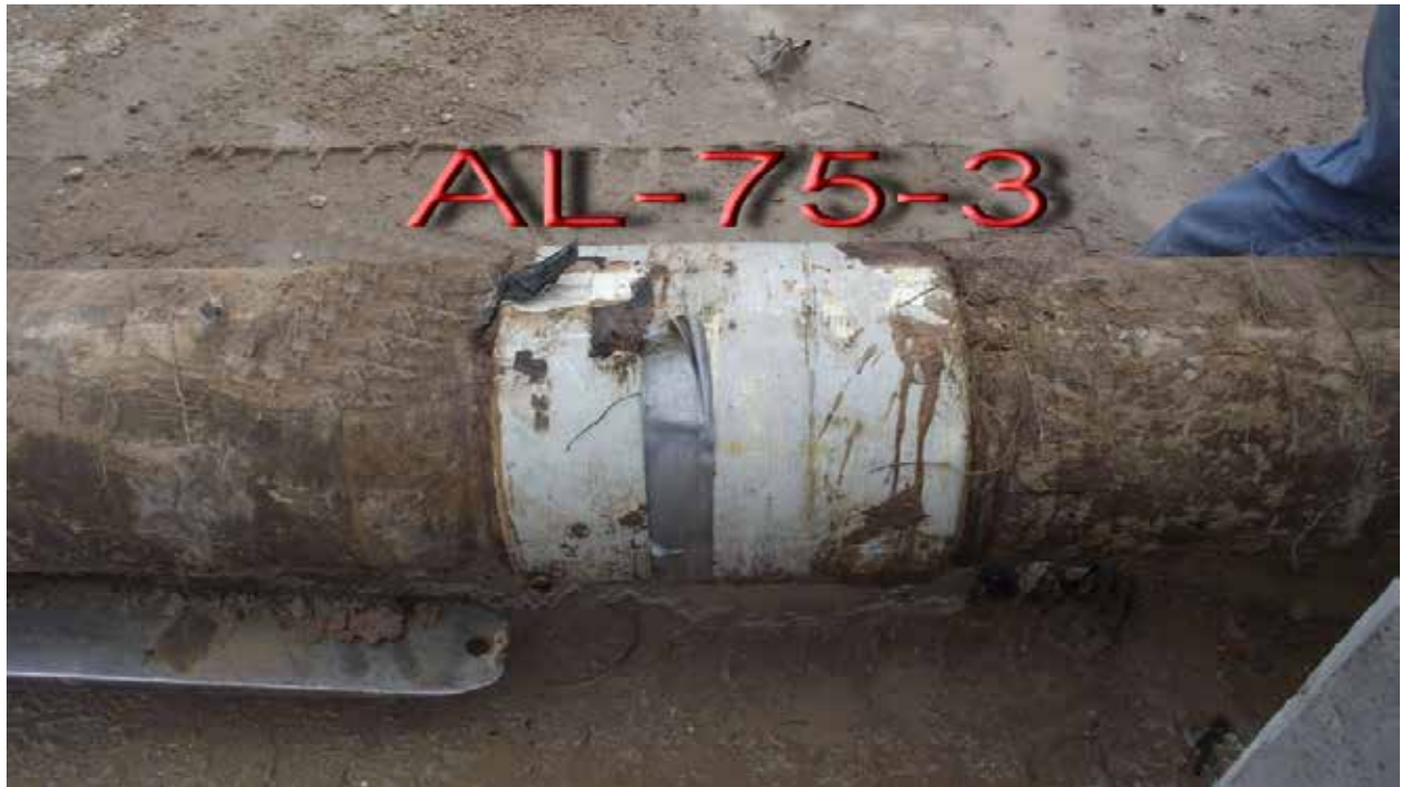
Figure 6 – Photograph of Failure Location, 75% Corrosion Sample
