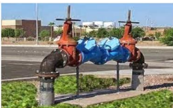
A commonly used valve to control waterflow to a fire sprinkler system is known as an
