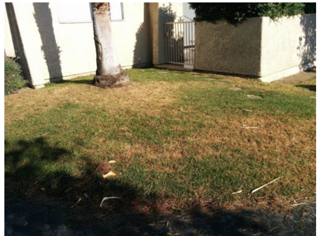
Grass is brown here because the sprinkler is blocked by the palm tree. This is an area where a small amount of turf removal would be beneficial.
