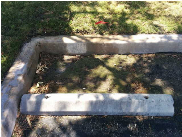
This sprinkler has been broken a long time, there is a thick layer of moss growing in this corner.
