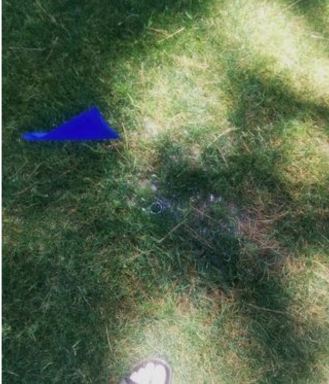
Broken sprinkler, doesn't pop up
