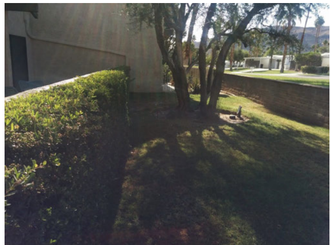
The location of the leak
