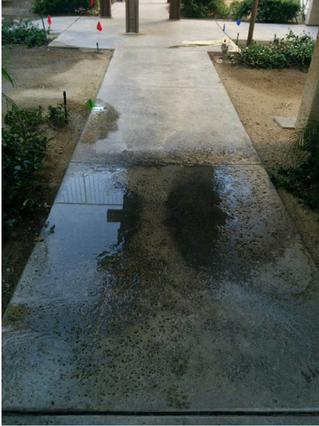
A lot of overspray and slippery concrete
