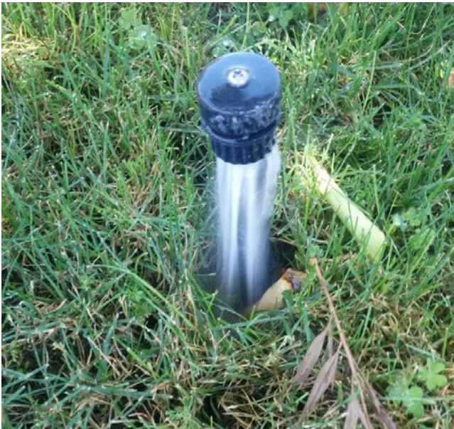
Why we don't leave equipment in place if we're not using it. They fail and no one notices.
