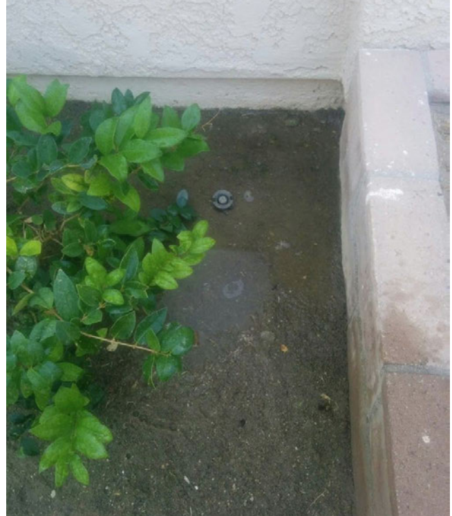
Another form of broken sprinkler, leaking
