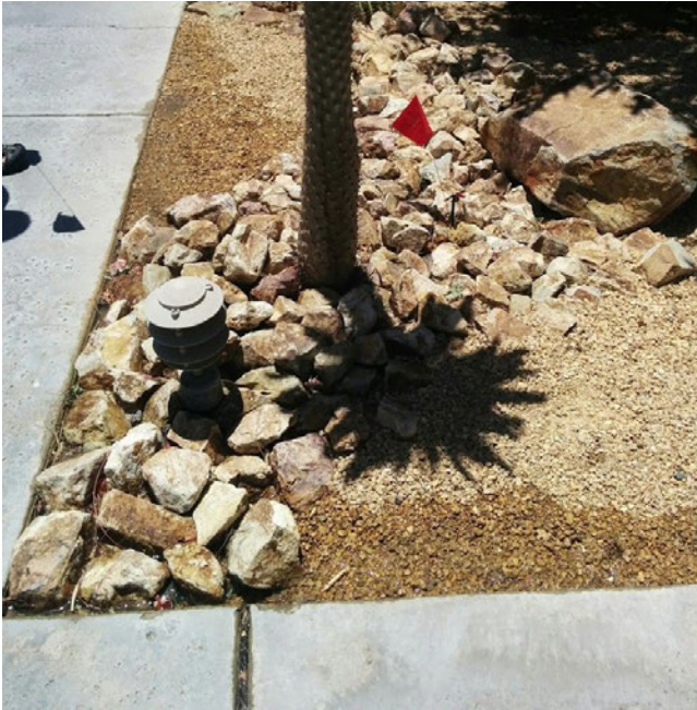
Water is pooling in the desertscaping from a broken emitter.
