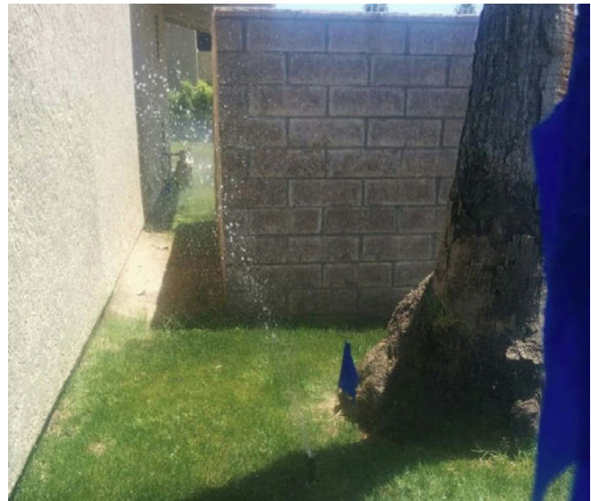
One of many sprinklers that were broken and would be detected with regular wet runs.
