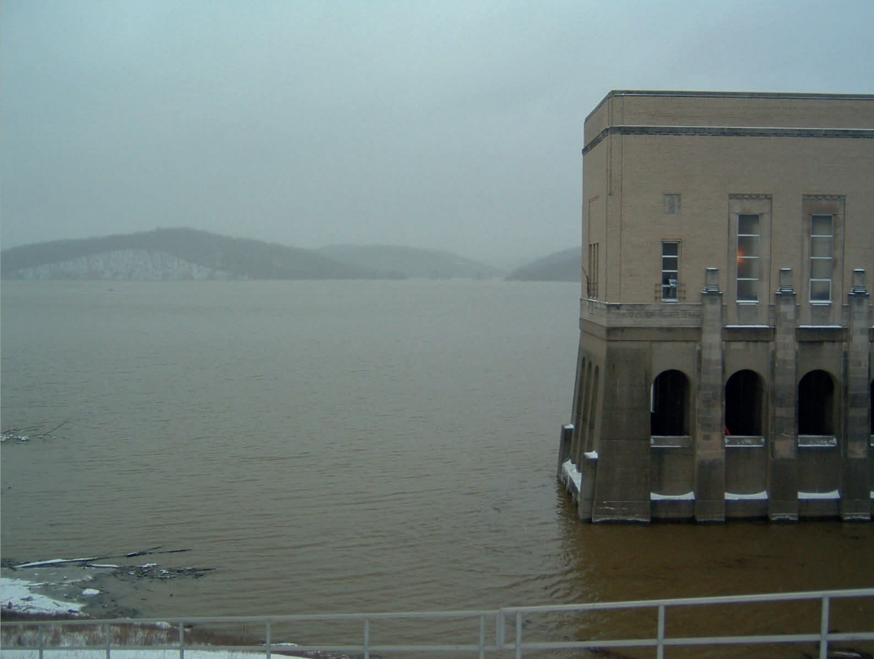
Mohawk Dam on the Walhonding River in Coshocton County, Ohio, USA during the January 2005 flood. Photo credit USACE
