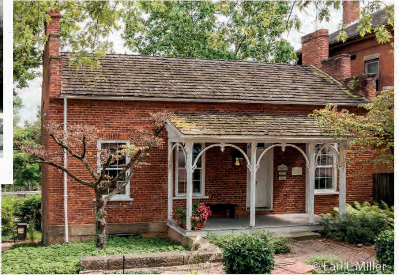
Roscoe Toll House before and after. This was the first building Montgomerys restored. Photo credits: See photos.
