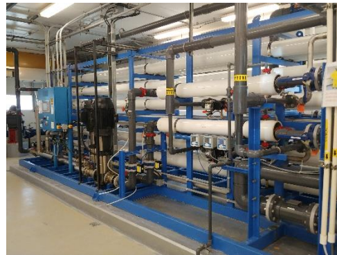
Reverse Osmosis Filters and Lines
