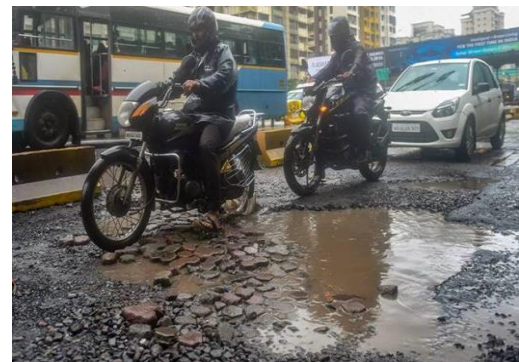
Figure 2: Condition of roads with potholes.
