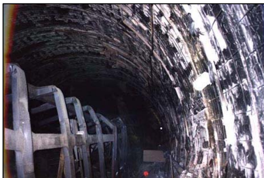
CHANNEL TUNNEL FIRE 1996 – EXTENSIVE CONCRETE LINER DAMAGE
