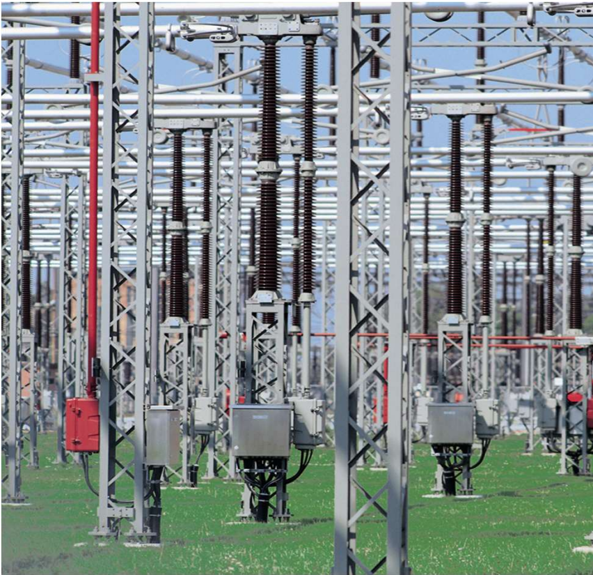
Transformer substation switchgear
