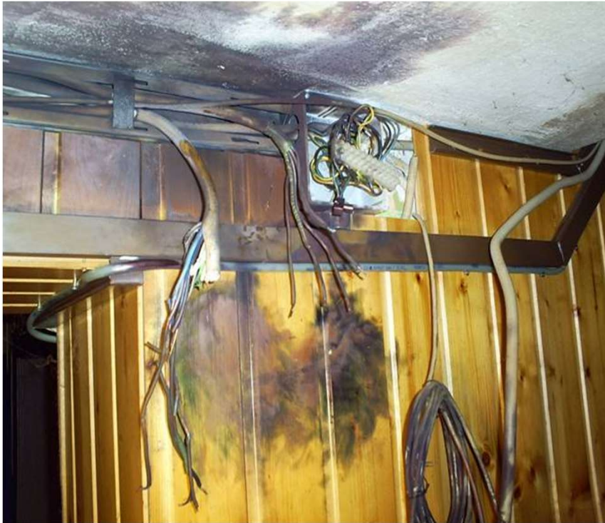
Junction box first floor
