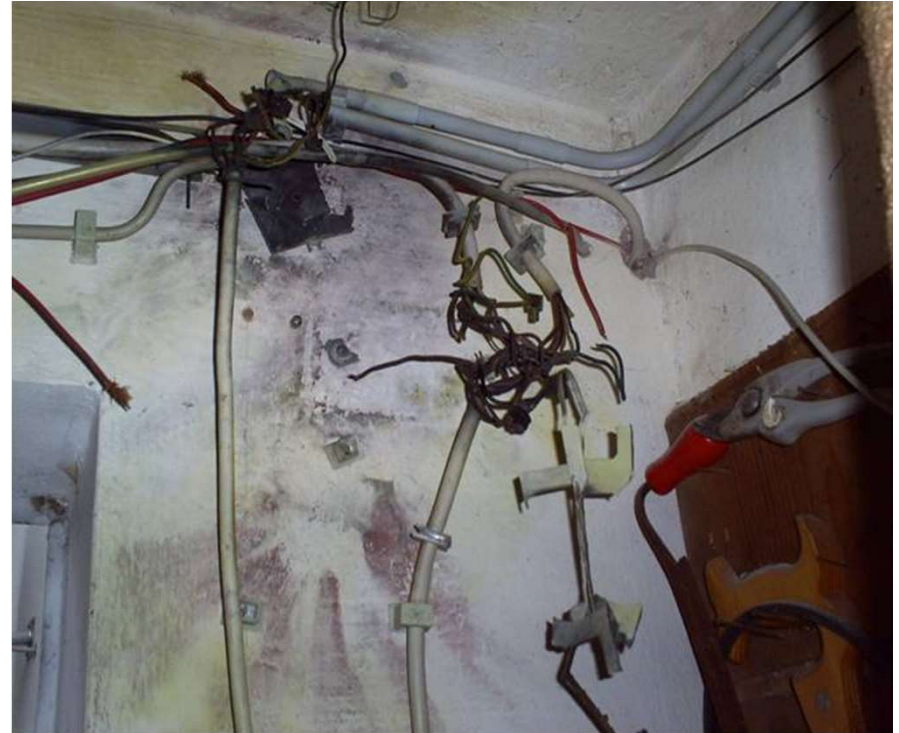
Junction box basement
