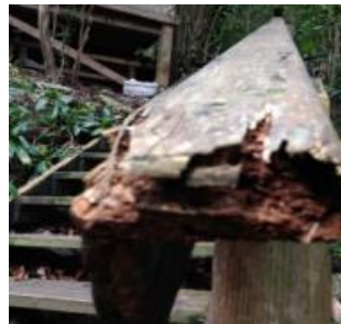
Railing replaced in 2011 already rotting while stairs from 1983 still sound.
