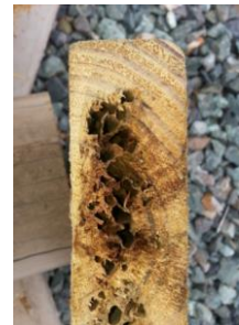
Termite damage difficult to recognize from the inside out
