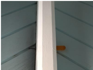
Screwdriver pushed through a dry rotting interior structural roof rafter beam.
