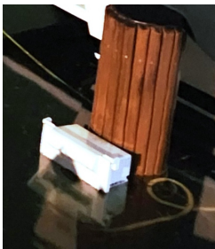
Submerged dock power pedestal
