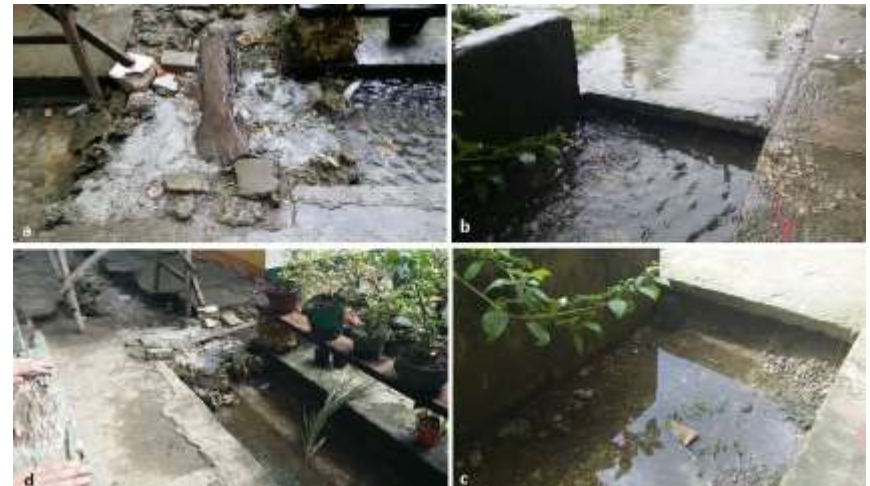
(a) & (b) Drains clogged with accumulation of water after rain.
