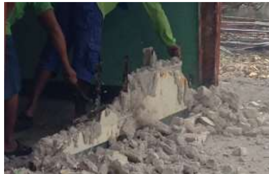
Little or no reinforcement found in existing structure
