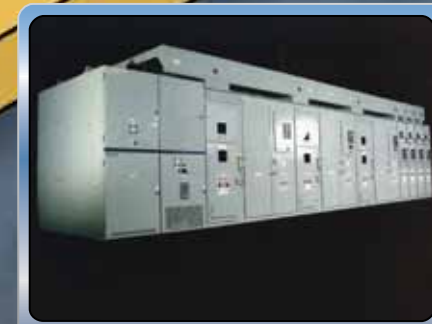
Motor Control Centers
