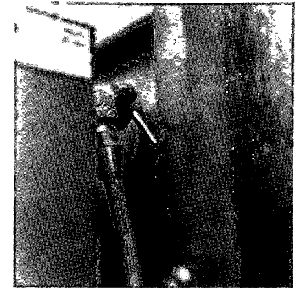
Furnace Gas Valve
