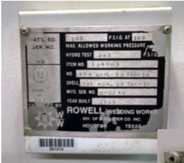
← Data Plate on Free Standing DDC Built 1985 by Rowell Welding
