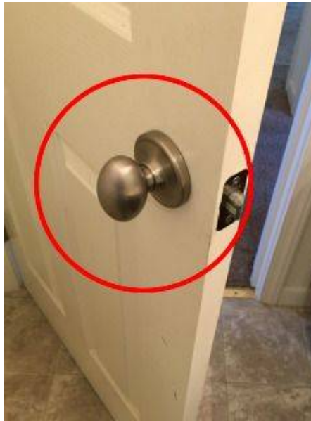
Photo 35-2 No Bathroom Door Lock
