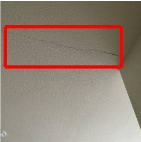
Photo 34-3 Ceiling Drywall Crack 2
