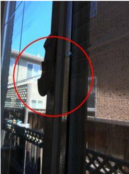
Photo 37-1 Kitchen Window Lock Faluty
