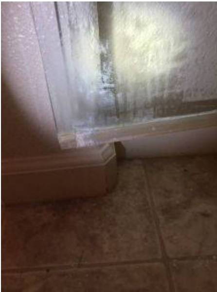
Photo 29-1 No Evidence of Tempered Glass
