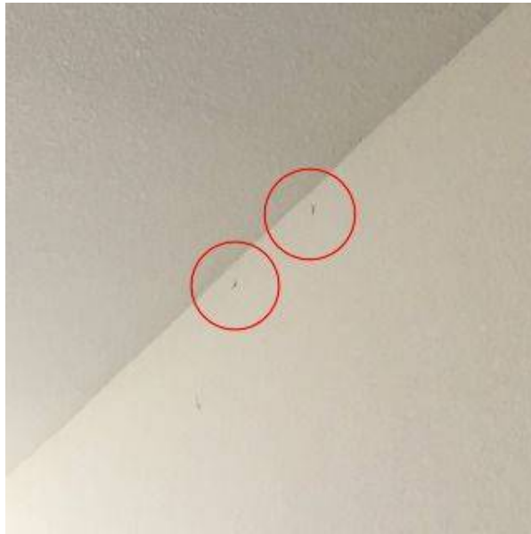
Photo 38-2 Drywall Nail Pops
