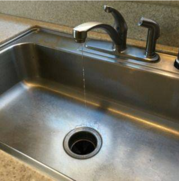
Photo 23-1 Dripping Kitchen Sink
