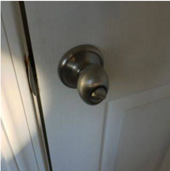
Photo 35-1 Faulty Bathroom Door Lock
