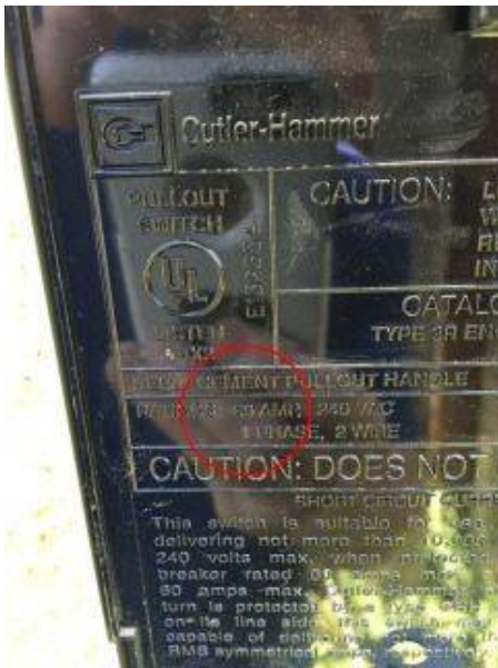
Photo 19-1 AC Disconnect 60 Amp Rating
