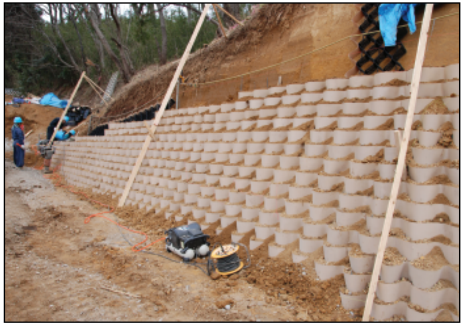
Precision Japanese construction ensures exacting wall alignment and setback. Native infill soil eliminates the expense of importing soil.
