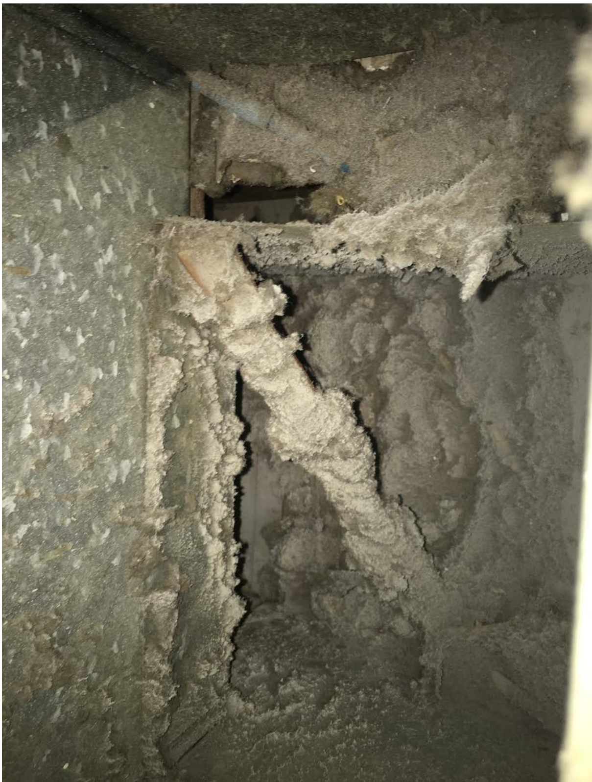
Figure 7 - Apartment 808 B Ventilation Duct
