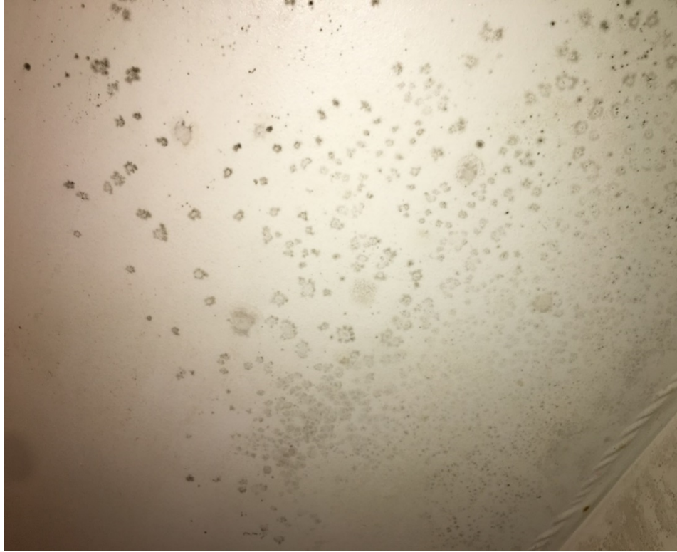
Figure 4 – Mold on the Bathroom Ceiling of the Smith Apartment
