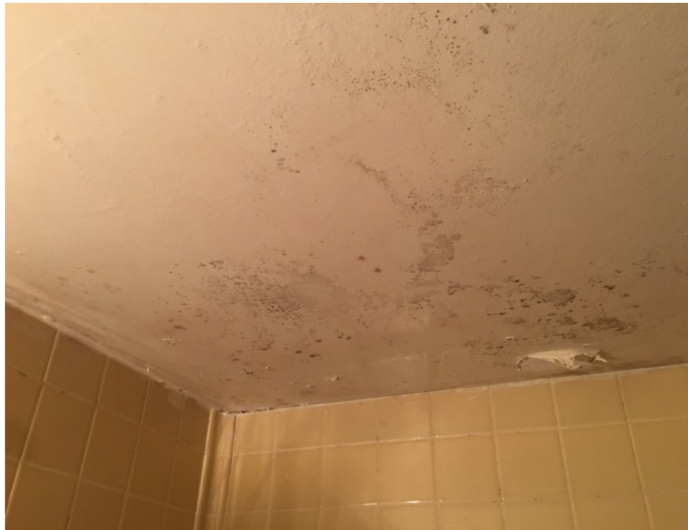
Figure 5 – Mold on the Bathroom Ceiling of the Smith Apartment
