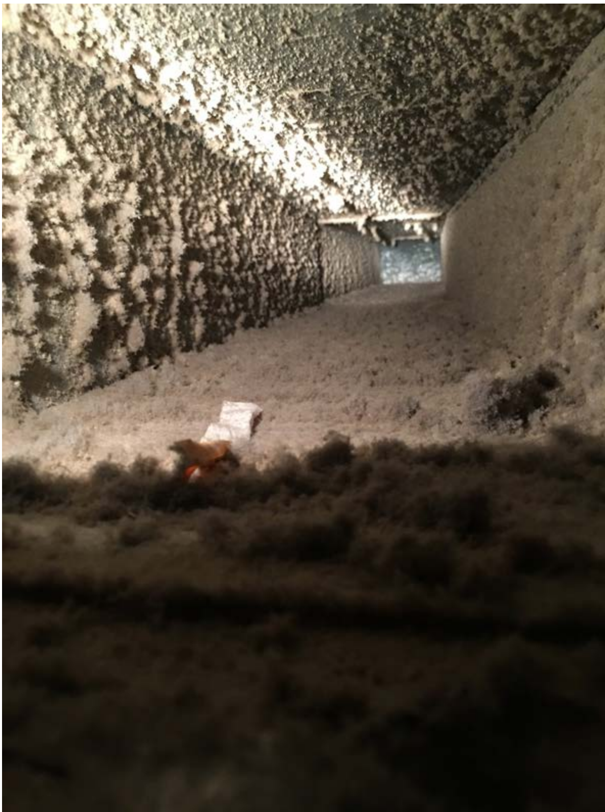
Figure 2 - Apartment 813 A Ventilation Duct
