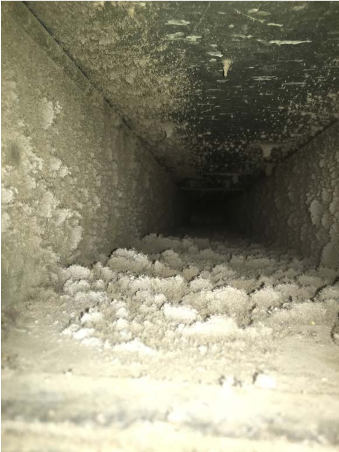
Figure 3 - Apartment 813 B Ventilation Duct
