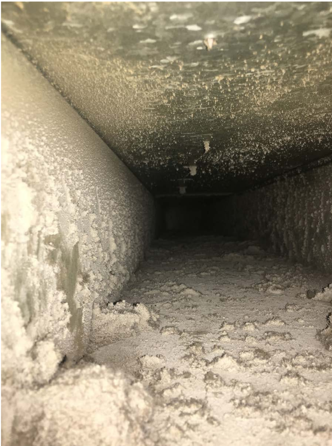
Figure 8 - Apartment 808 B Ventilation Duct
