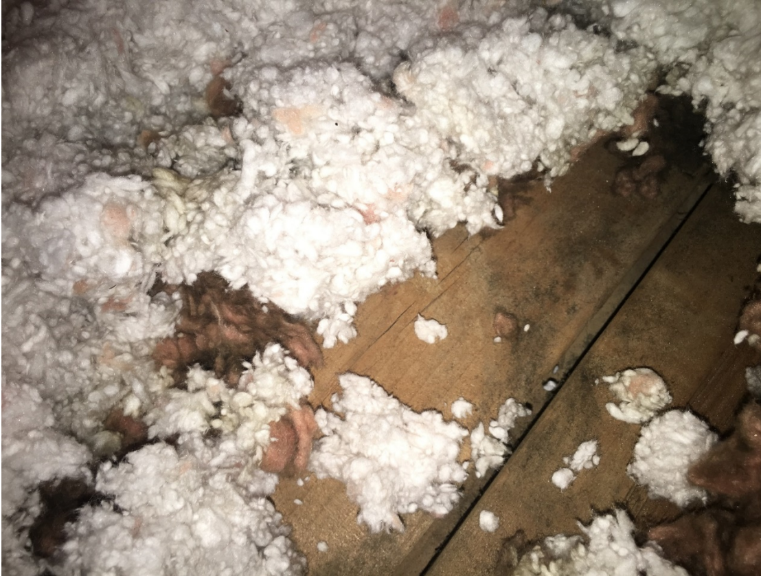
Figure 6 – Black Mold in the Attic immediately above the Bathroom Ceiling that was not remediated, but instead sealed into the Attic in the Smith Apartment days after this photo was taken.
