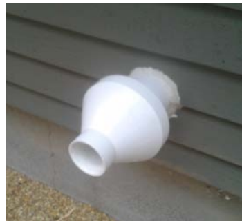
Wrong Vent Cover
