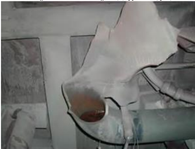
Figure 2: A valve operation in Hamaoka, Japan autoignited hydrogen and caused a piping explosion in a 6 inch diameter, ¼ inch thick steel pipe. Smaller explosions continue to occur in the U.S. reactor fleet and throughout the world (Appendix A, p. 9).
