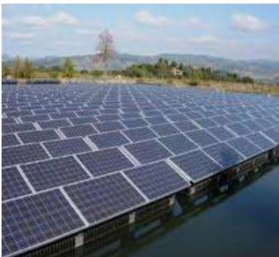
COMMERCIAL SOLAR PLANT
