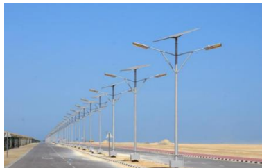
Solar PV LED Street Lighting
