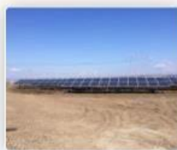
Reci, Covasna, RO 2,133 MW
