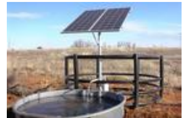
Solar PV Water
