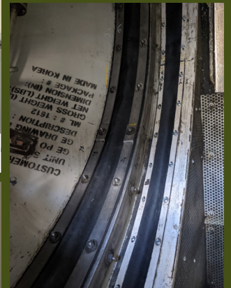
Bellmouth Seals Splice Area
