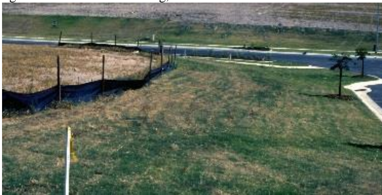
Fig.8 Use of a sediment fence and grassed strips on a development near Sinnamon Park, Brisbane Managing erosion in urban areas
