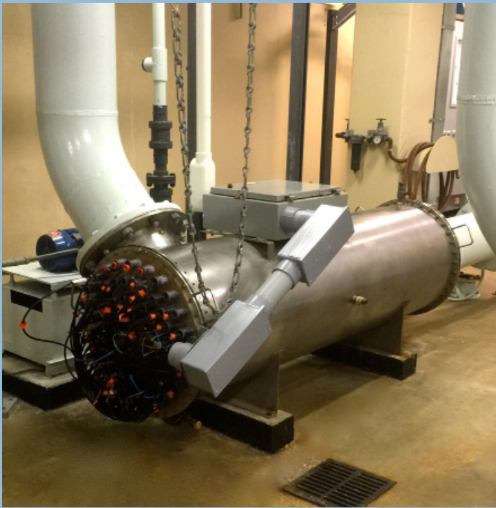
Old 316L chamber in excellent condition after 30 years held 72 low pressure lamps.
