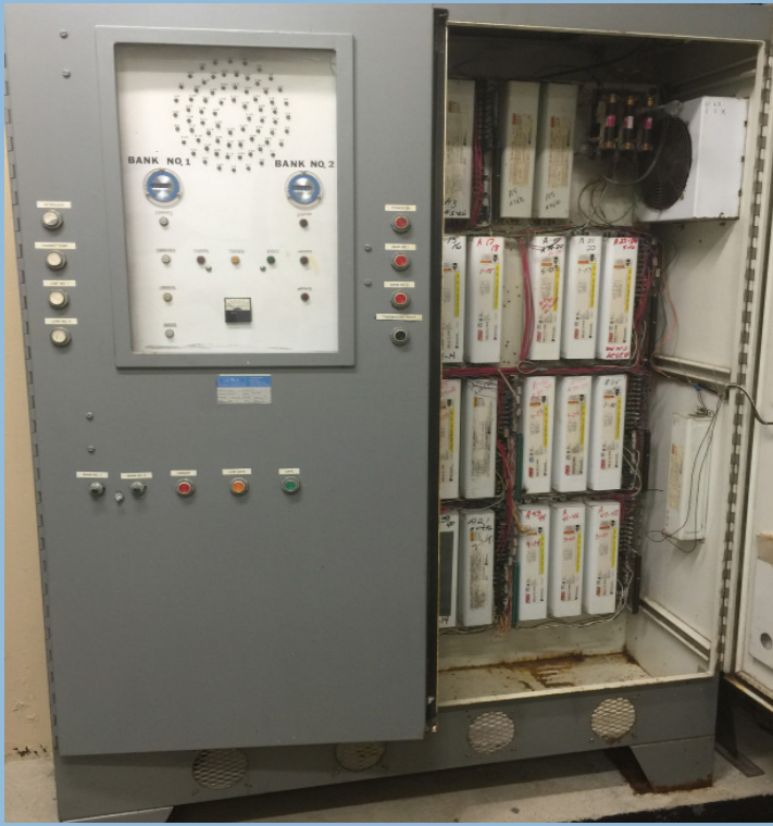
Old free-standing electrical enclosure with 36 magnetic ballasts.
