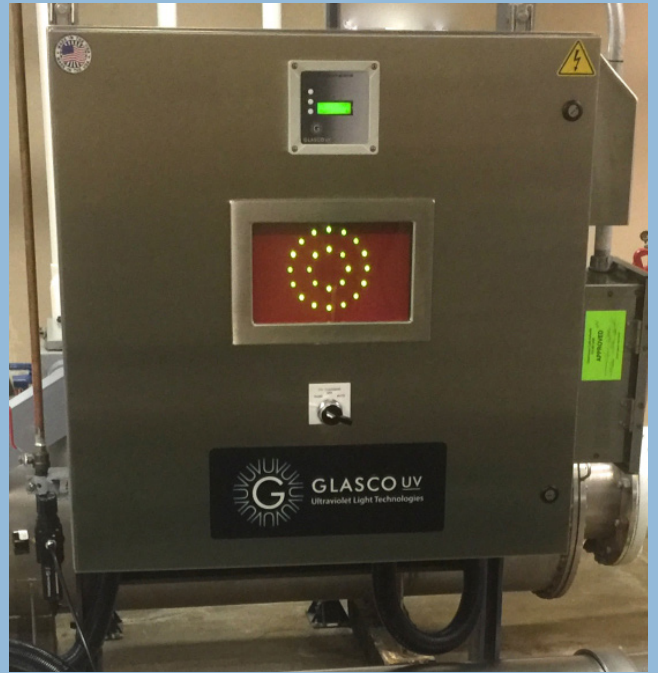
New wall-mounted electrical enclosure with electronic ballast
