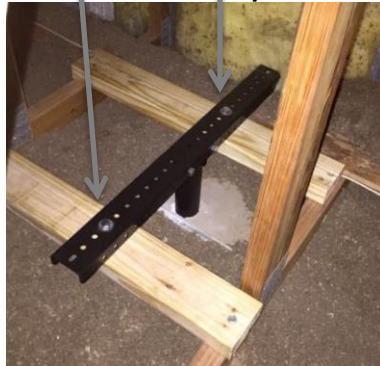
Bolt channels to support structure.
