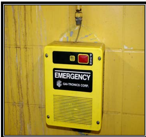
Figure 11. Call box with exposed wire
