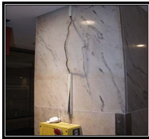
Figure 12. Call box with exposed wire
