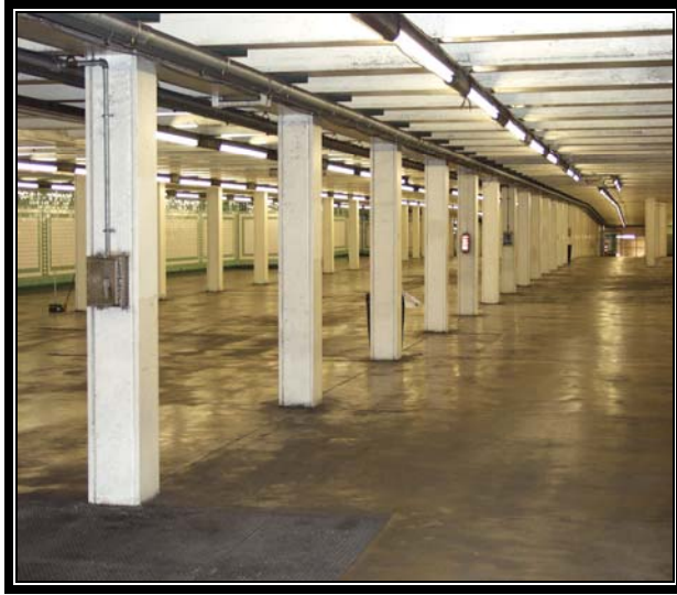
Figure 13. Emergency phone is mounted on the 5 th pole. Plumbing fixtures are mounted on the 1 st and 7 th poles.
