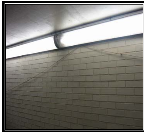
Figure 10. Dangling wire – no conduit
