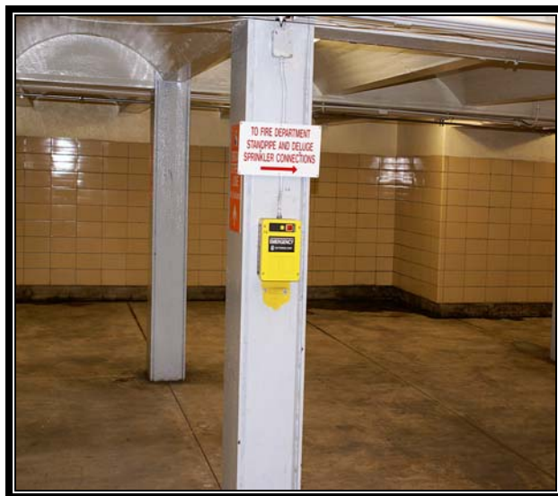
Figure 17. New box with no backing.
