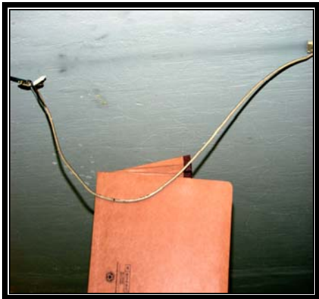
Figure 9. Dangling wire – no conduit
