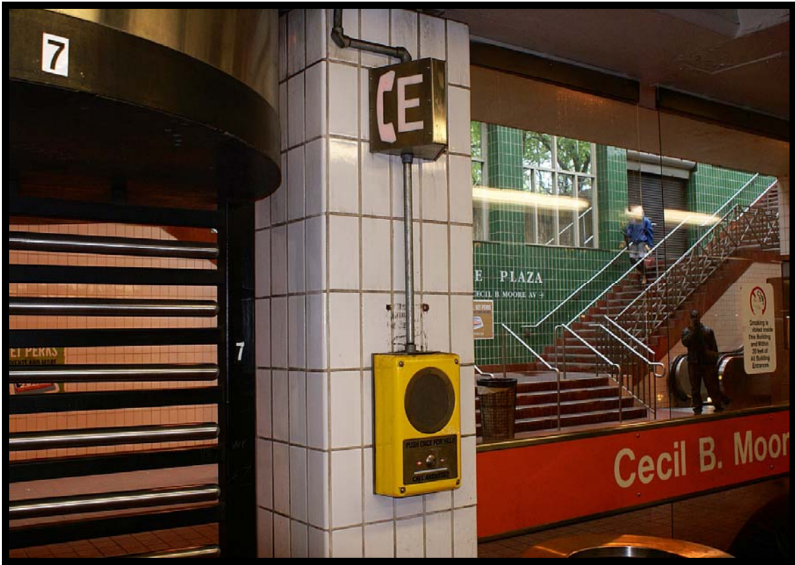
Figure 22. SEPTA call box. Note announcement light and metal conduit.
