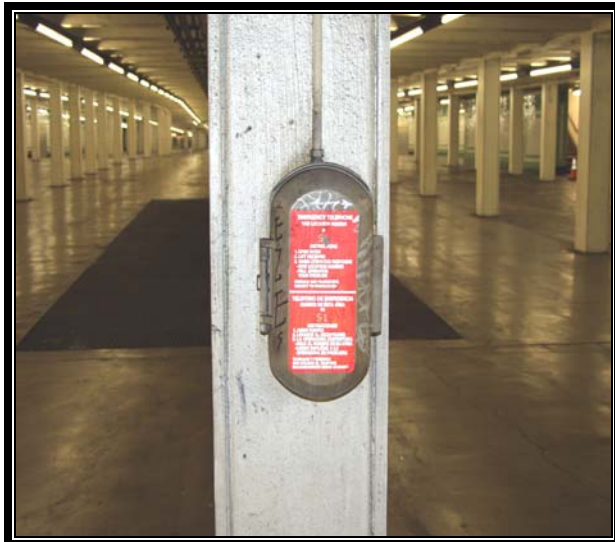
Figure 14. “Emergency” label is illegible, even from this distance.
