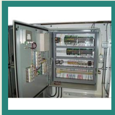
Motor Control Enclosure
