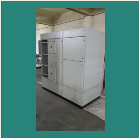
Industrial Control Enclosure
