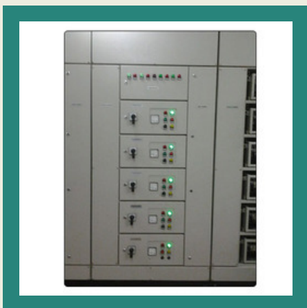
GA Standard Single Front Drawout MCC Panels
