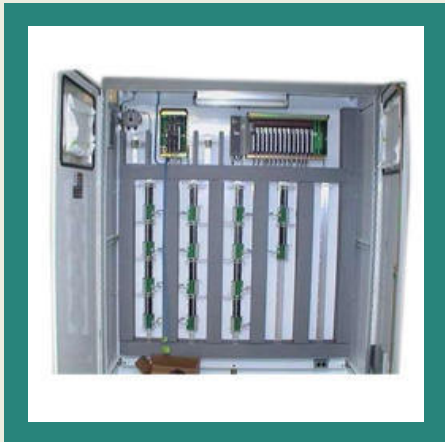
Marshalling Panel Enclosures
