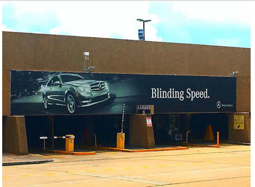
TS32 - One of the eight 9 ft x 72 ft frames installed at the Mercedes Benz Superdome New Orleans parking entrances. The frames and graphic installation with white inserts fixed on the side of the frames was realized by CC Imaging.
