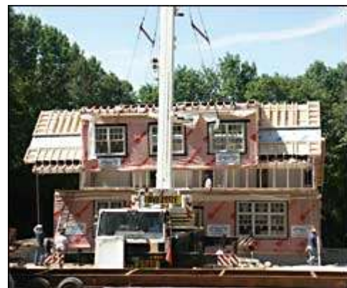
All in a day's work. In just a few short hours, the bare foundation now supports an almost complete home.
