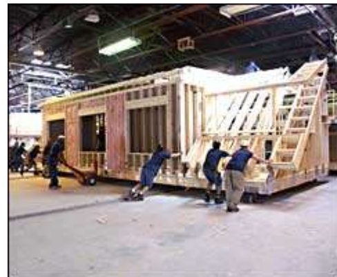
Workers maneuver a section of a house into position for additional assembly work.
