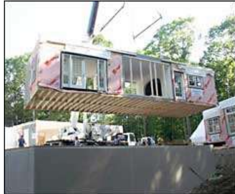
Direct from the factory. The first section of the house is lowered onto the foundation by a crane.
