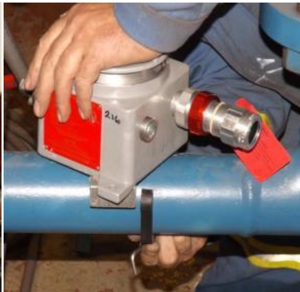
Exp. Proof Box being clamped onto Pipe Note: Explosion Proof fitting for Haz. Loc.
