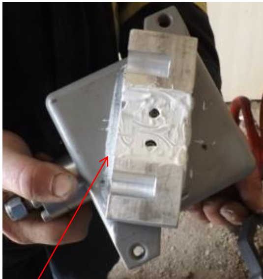
Thermal Grease between Explosion proof box, saddle clamp, and between the saddle and pipe.
