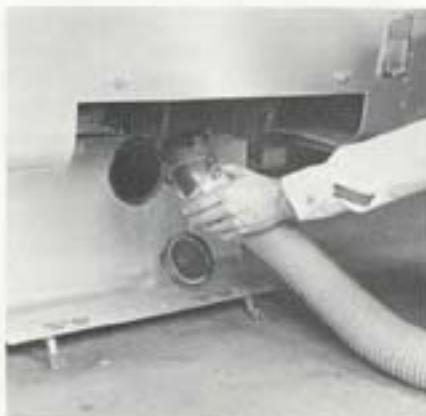
Sewage Hose Connection
