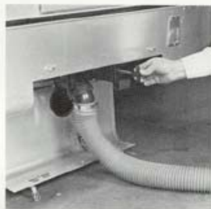
Waste Holding Tank Drain Valves
