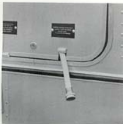
City Water Connection
