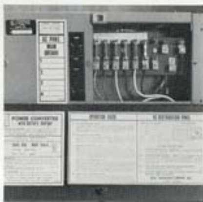
Electrical Control Center
