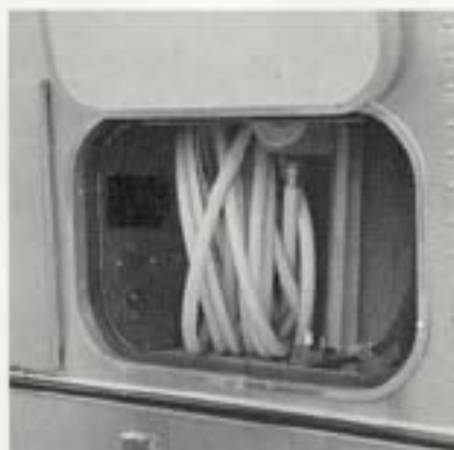
Cable TV Terminals
