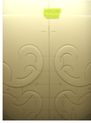
The PerfectaStripe curve template is now aligned with the vertical centerline. Desired curves are transferred. The template is then repositioned and additional curves are marked.
