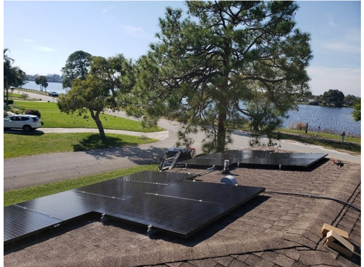
Solar panels facing the sunny side
