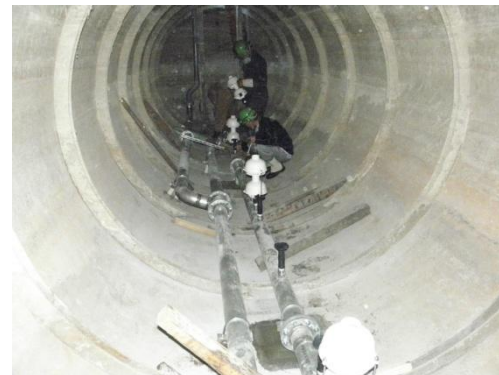
Inside of aeration tank
