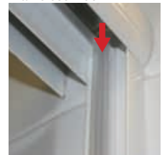
Watertight Seal on Wall Channel
