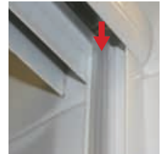
Watertight Seal on Wall Channel
