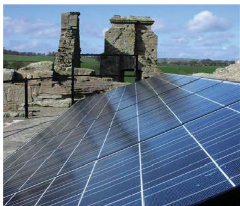
PV installation on a flat roof at Crichton Castle, which is now in the care of Historic Scotland (Photograph courtesy of Historic Scotland)
