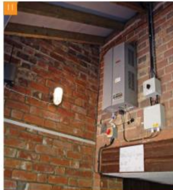
11 An installation, showing the inverter, isolator. (Photograph courtesy of Solar Century)
