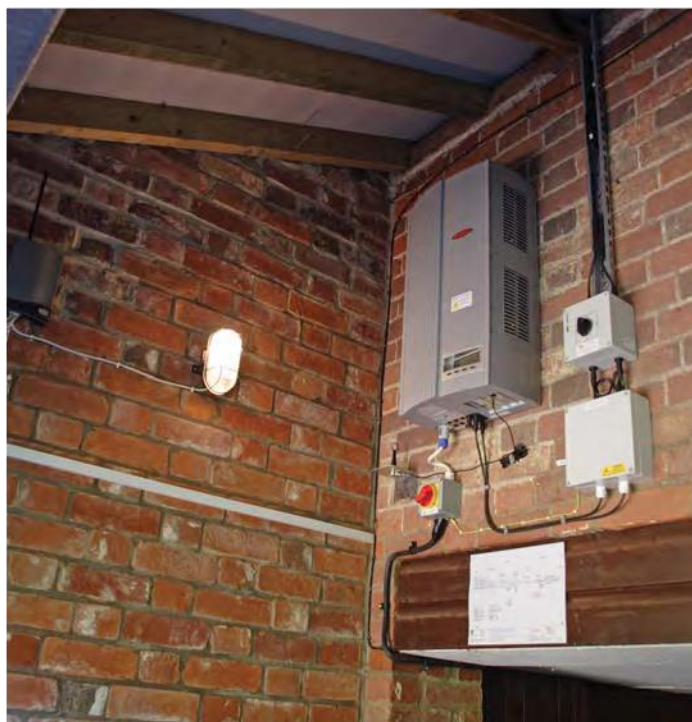
Typical Inverter installation
