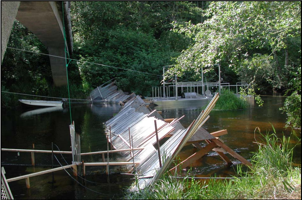
Figure 5.25. Photo looking from the right to the left bank of the Ozette River, showing the counting weir, adult trap, and rotary screw trap.
