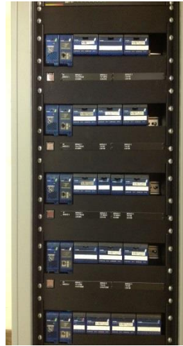
Factory Assembled I/O Module Strings Located In Right Hand Bay Module Door
