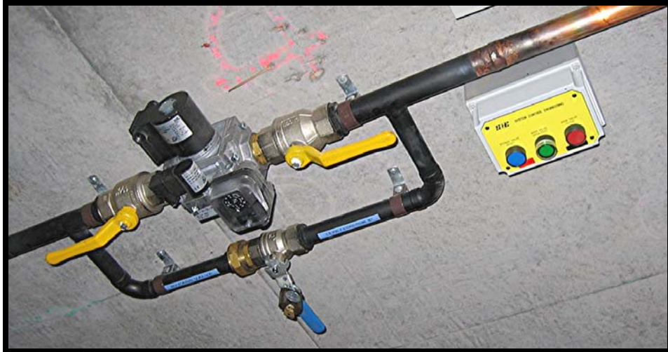
Figure 1 – Gas Shutdown System
