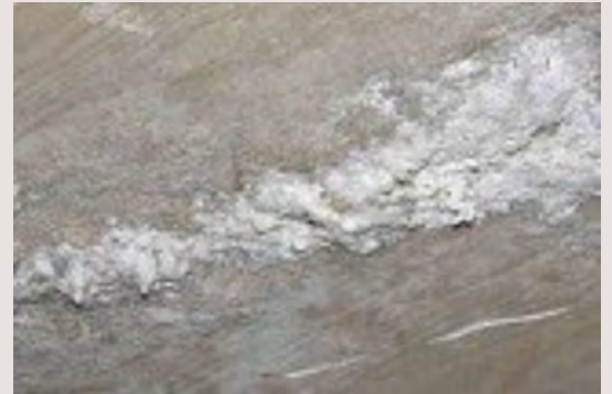
Example of secondary efflorescence in parking garage exposed to diluted road salt from vehicles entering the garage during winter.
