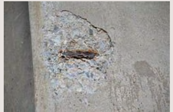
Example of flat piece of concrete having dislodged with corroded R-bar underneath.
