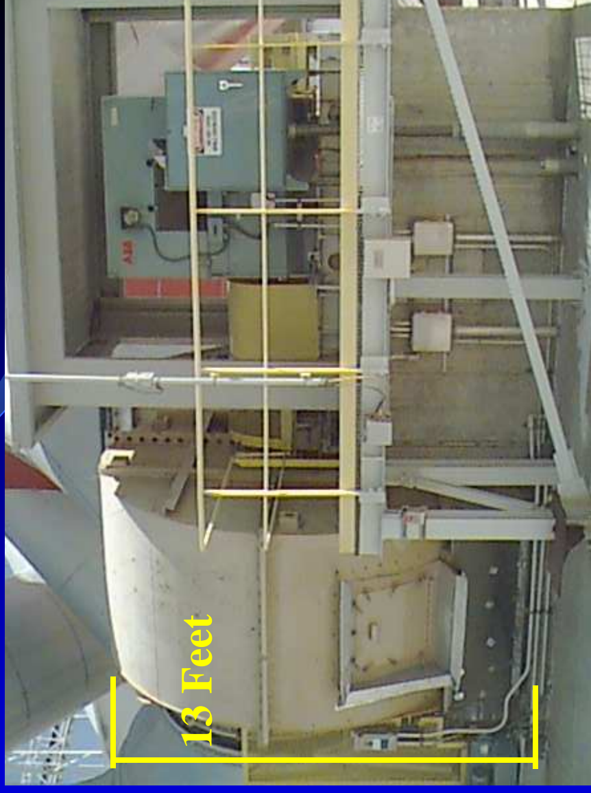
Illustration A. Overview of Scrubber Fans Evaluated 11B-4
