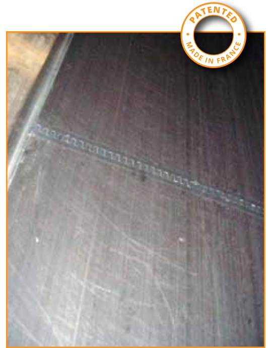
PVC splice at an airport baggage carousel
