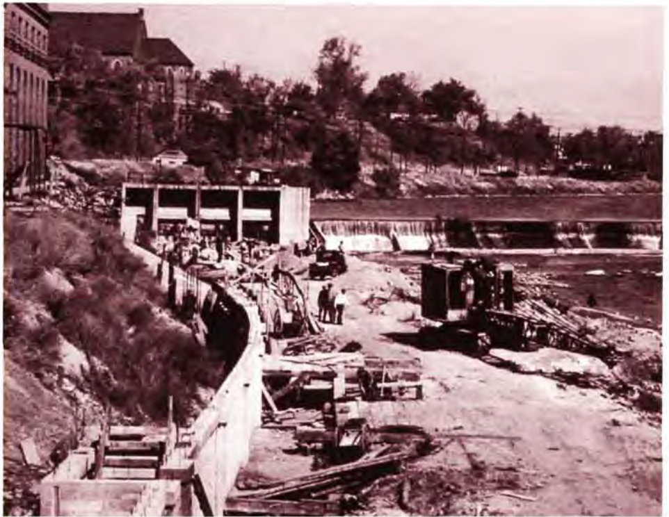
W.P.A. construction of the west river wall along the Des Moines River, 1939
