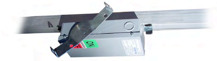
Fused Disconnect installed on STARLINE
