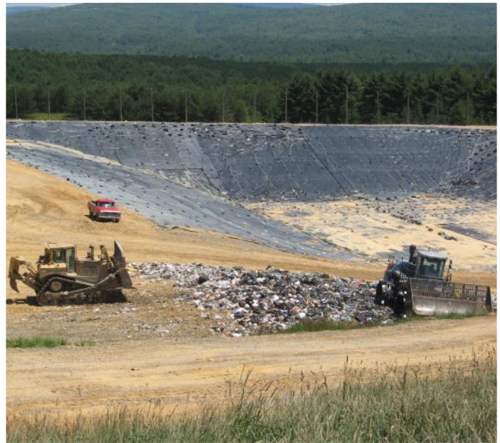
Tucker County Solid Waste Authority Landfill is located between Davis and Thomas, West Virginia
