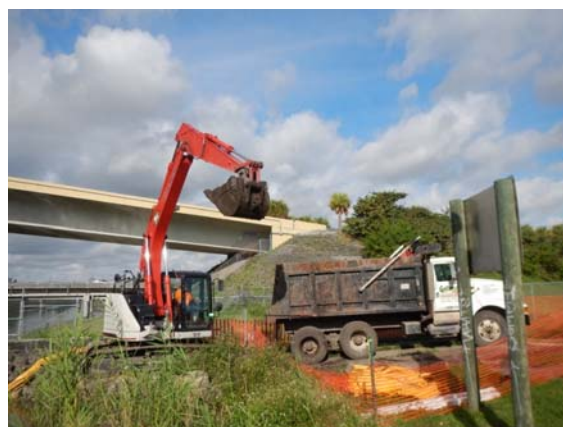
And into the dump truck, to be hauled to the landfill site.
