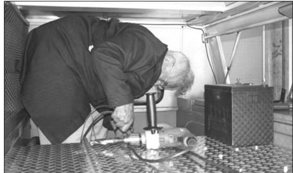
Paul Kydd gets set to install another battery inside the rear cab of the S-10 Chevy pickup.
