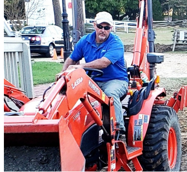
Scott Chandler at work on our latest service project to construct a ramp to the Carriage House of the Watermen's Museum
