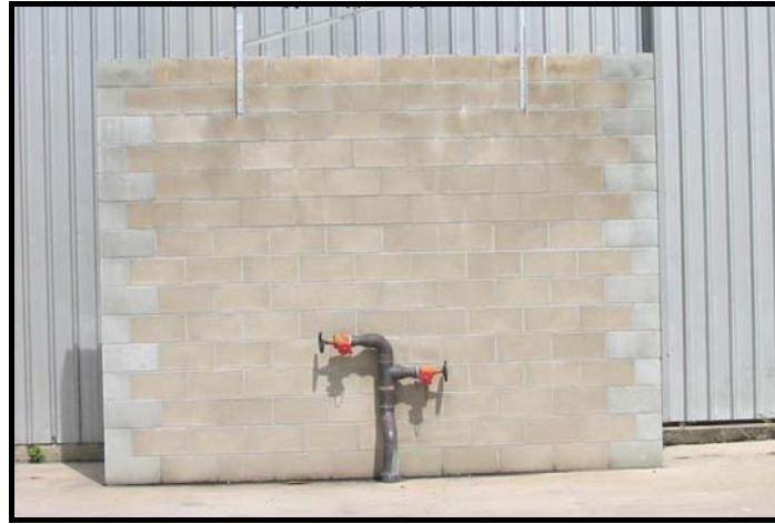
Figure 4 – Protection of External Hydrant
