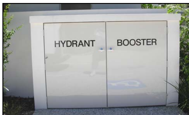
Figure 6– Stainless Steel Booster Cabinet
