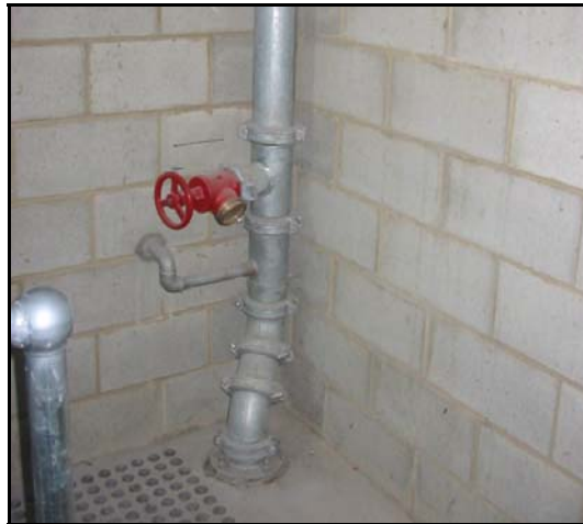
Figure 2 – Hydrant in Fire Isolated Stair
